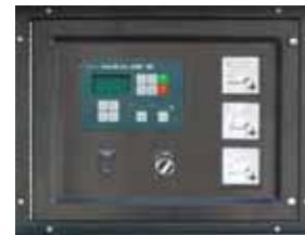
Control panel for soundproof
